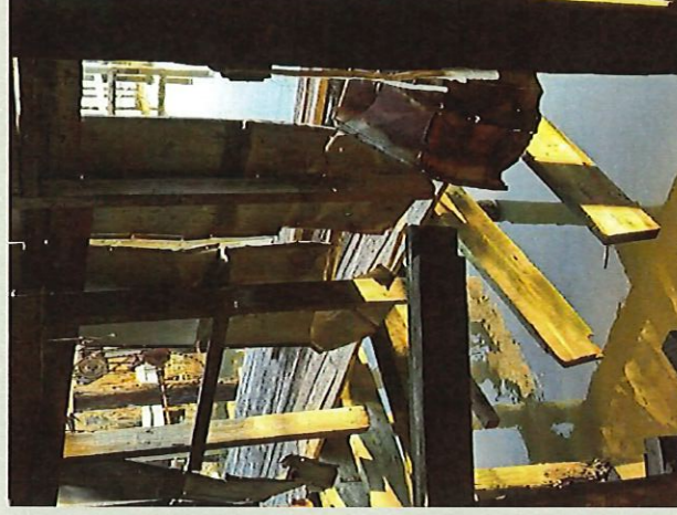
Illustrates floor damage
