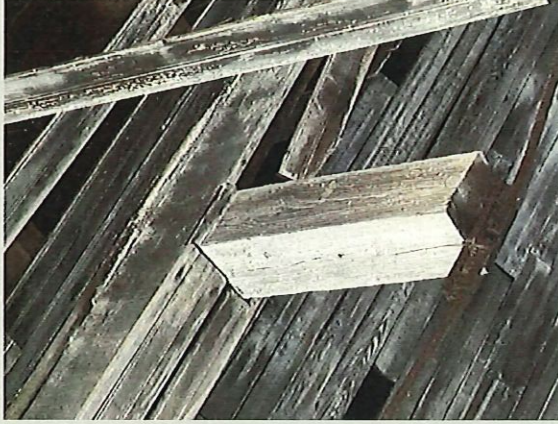
Column disconnected, being held by metal bar
