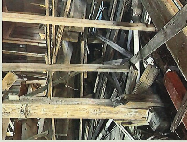
Illustrates floor damage
