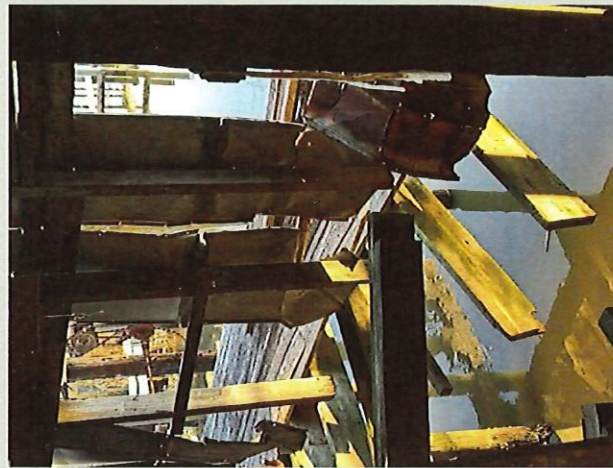
Illustrates floor damage
