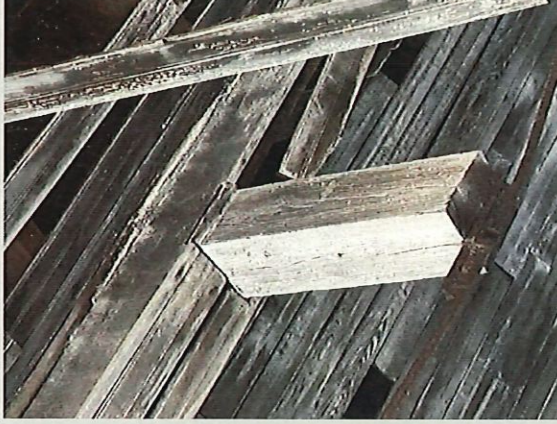
Column disconnected, being held by metal bar
