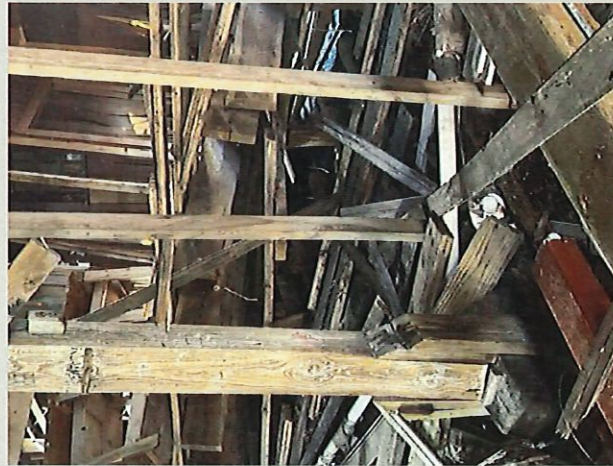
Illustrates floor damage
