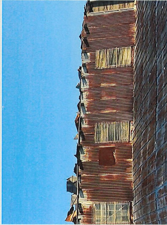
Roofing peeled back by Hurricane Michael around perimeter South Elevation
